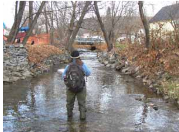
Figure 5.62: Straightened channel with bank armoring and lacking riparian buffers near the intersection of Traverse Street and Union Street
