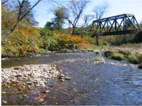
Figure 5.5: Diagonal bar, bank armoring and railroad bridge near where railroad crosses Route 12
