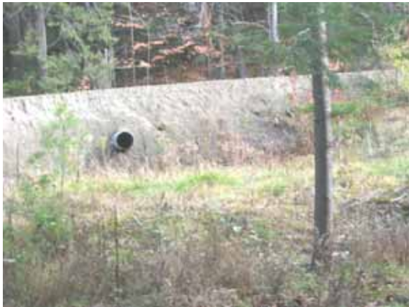
Figure 5.68: Stormwater outfall in loose road material that can easily wash into channel downstream of Stony Brook Road Bridge.
