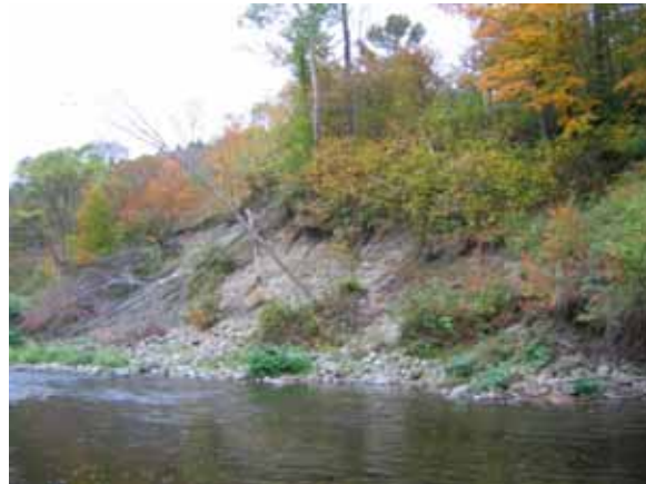
Figure 5.11: Mass failure on right bank where straightened segment begins downstream of Chase Brook confluence
