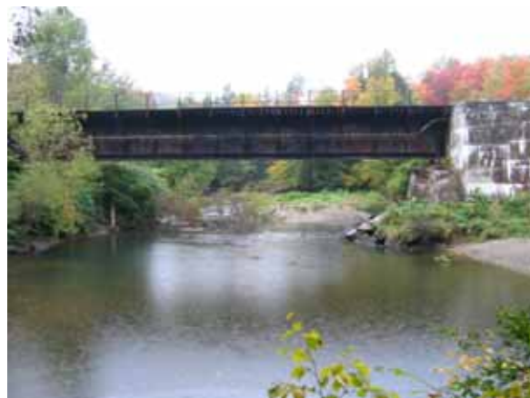
Figure 5.17: Large pool above waterfall and mid channel accumulation upstream of railroad bridge near Route 12 and Pine Hill Drive
