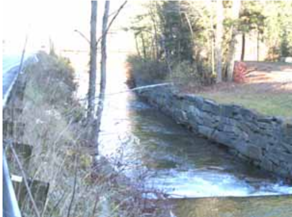
Figure 5.63: Straightened channel with armoring on both banks and small dam along Lovers Lane near the intersection with Route 12A
