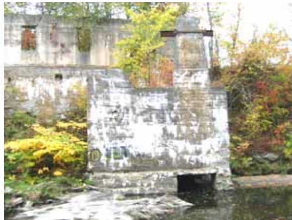
Figure 5.14: Old mill structure channel constriction downstream of Route 12 bridge near Berlin Volunteer Fire Department
