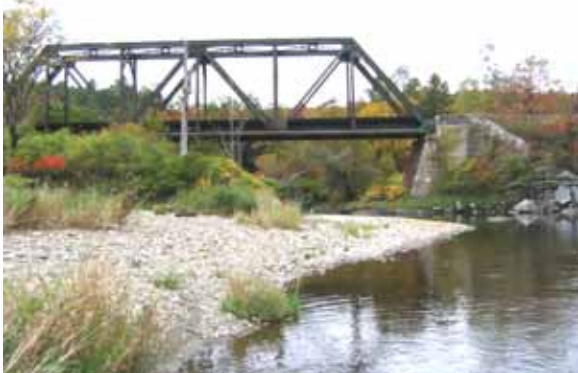
Figure 5.13: Mid channel accumulation below undersized railroad bridge near West Berlin Cemetery
