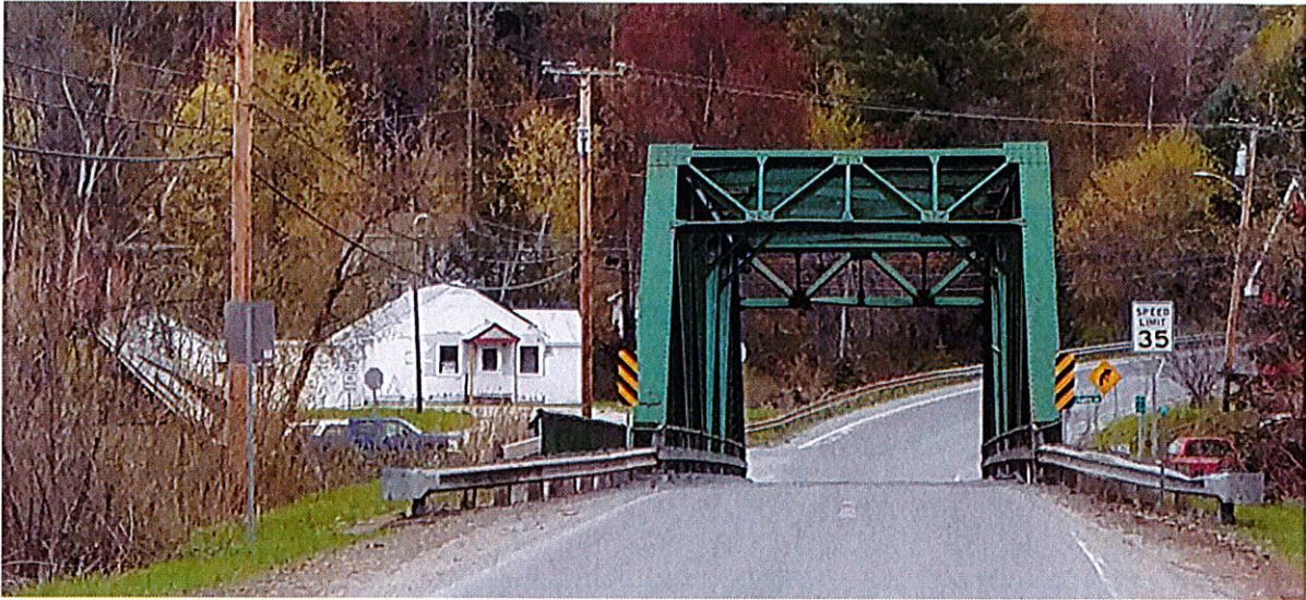
E. View of the bridge and the currently unused General Store (Building 12) from Route 12 looking east.
